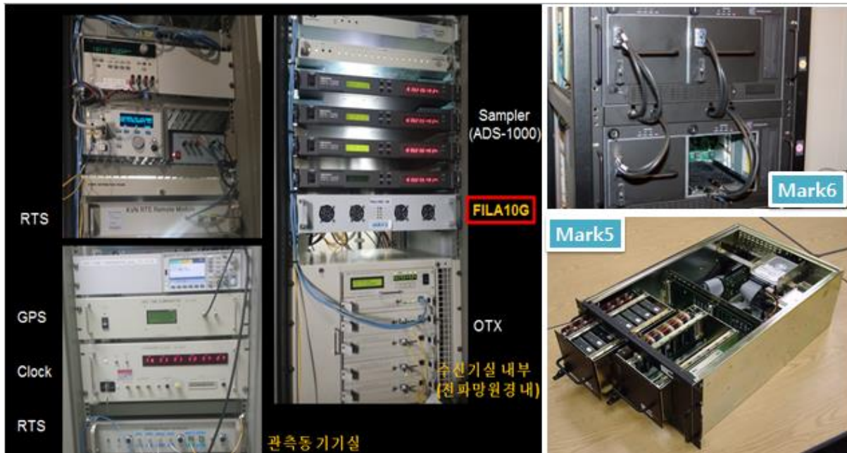
Figure 2. KVN data acquisition system with newly installed FILA10G and Mark6 systems.
